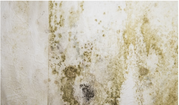
Typical example of mould growth on wall using incorrect plasterboard.
